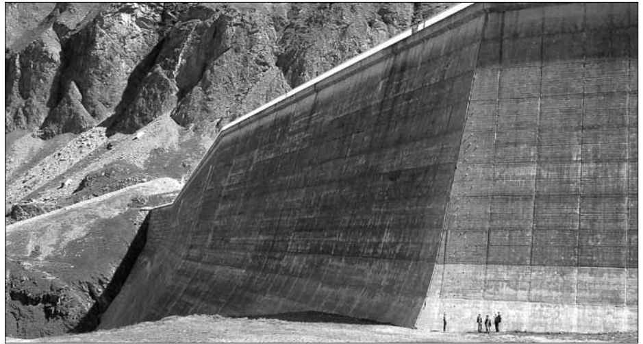
The dam wall of Grande Dixence, one of the biggest hydro power plants in Switzerland. (picture wikimedia/Paul Kordwig)
