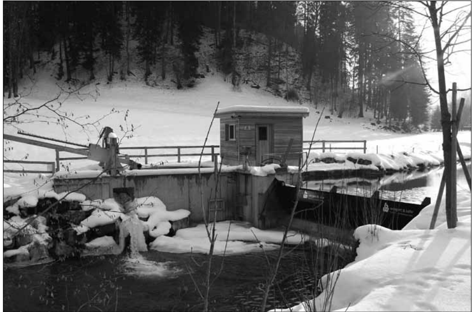
This miniature hydroelectric power plant supplies 70 households with electricity. (picture thk)
